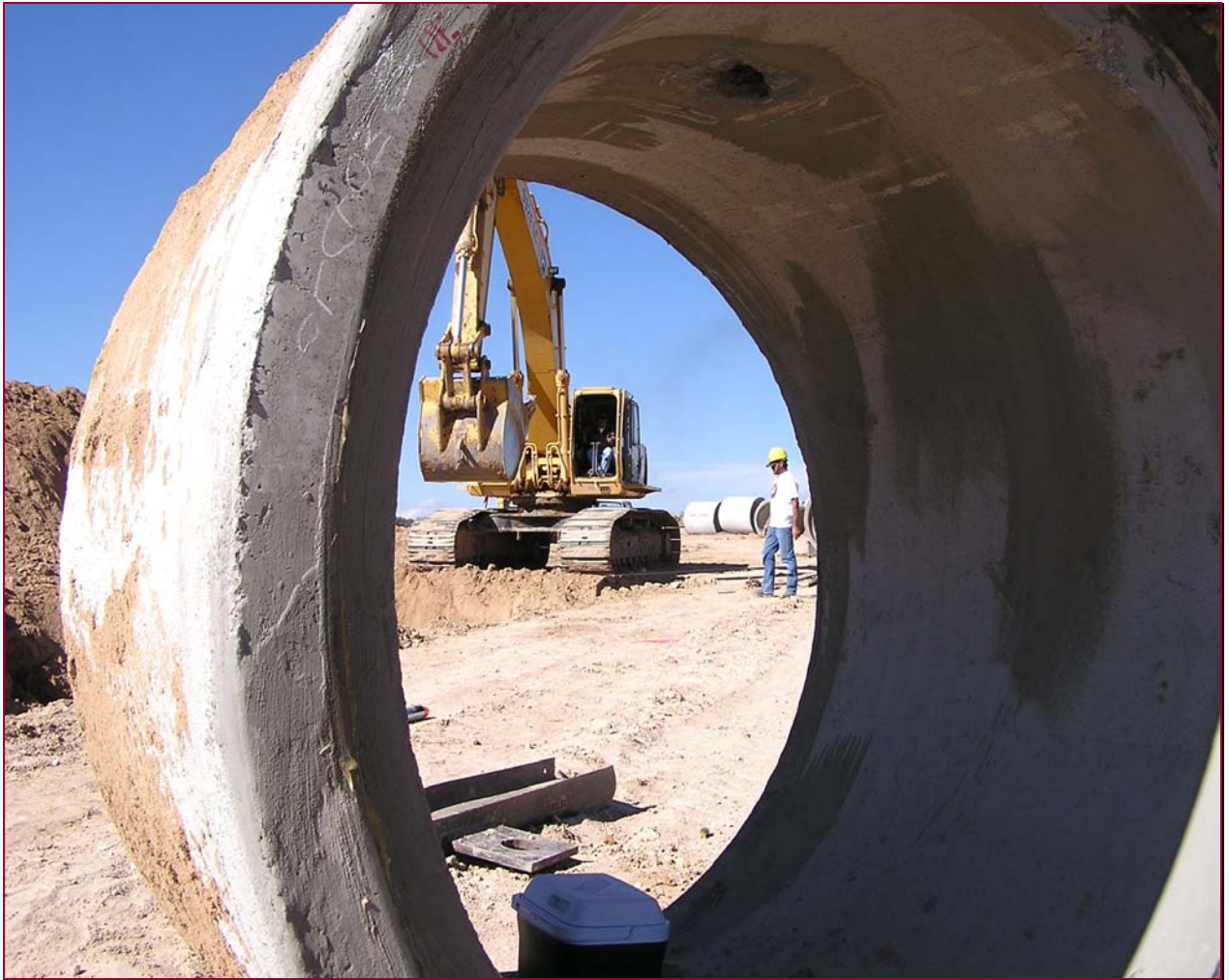
Placement of 72 inch RCP in Phase 1 of Phase 1 of Cabezon Development in Rio Rancho
