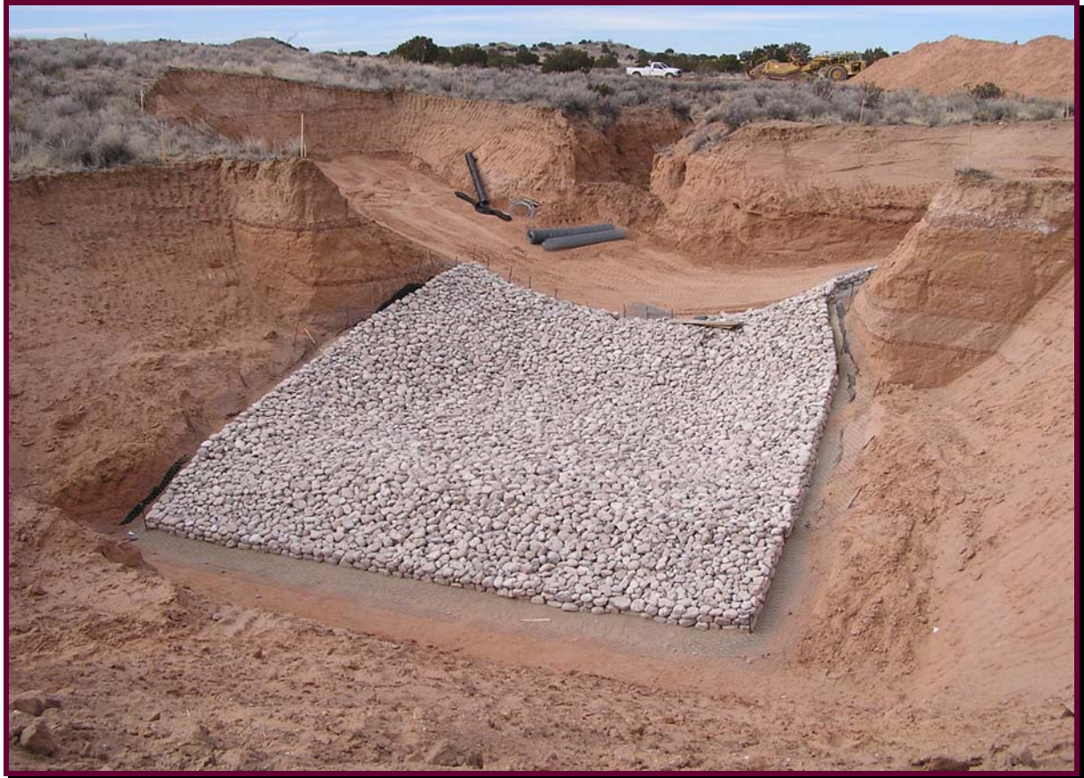
Rip Rap Drop structure constructed in the Venada Arroyo tributary in the Mariposa Subdivision
