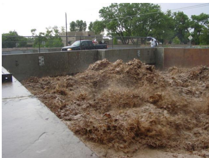
Figure 6: 2006 – Hydraulic jump occurring at Corrales Road bridge
