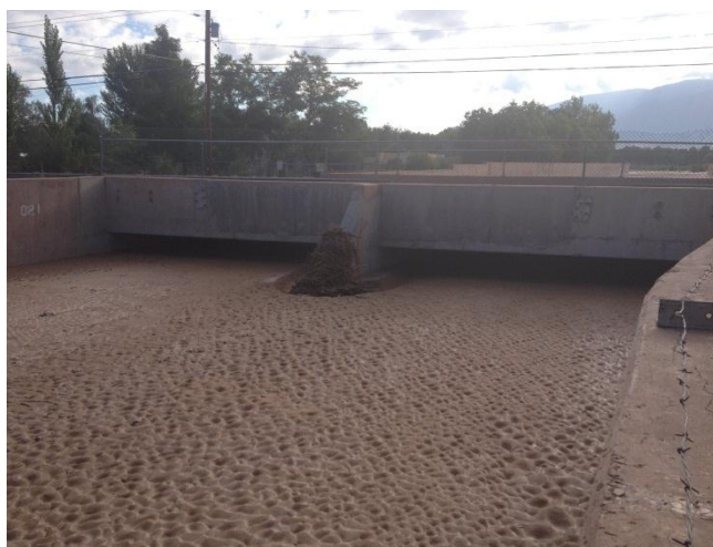
Figure 11: 2013 - Sediment deposition under Corrales Road bridge
