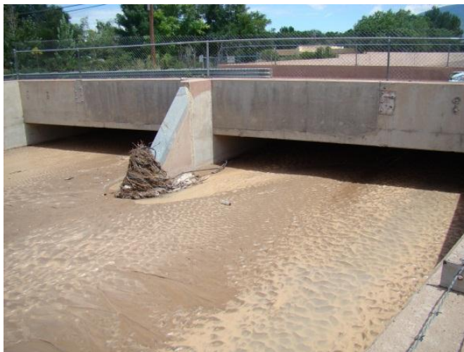
Figure 8: 2010 – Sediment deposition under Corrales Road bridge
