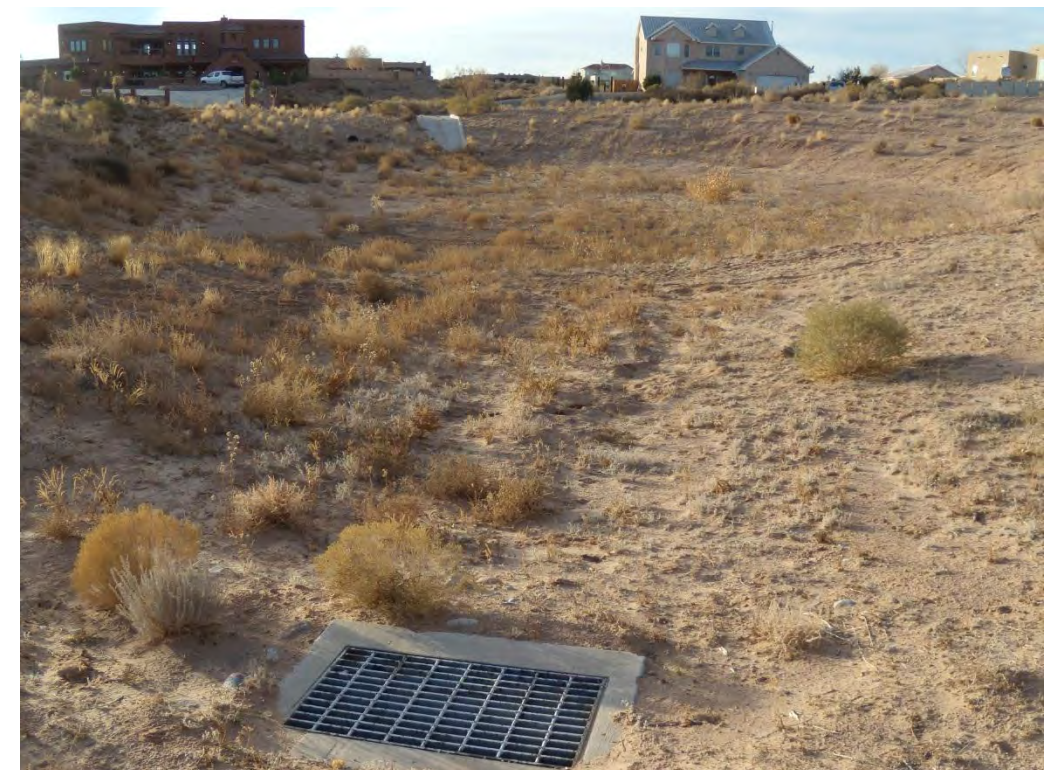
Photo 6: Christopher Pointe Pond (WC_06P, capacity \approx 2 AF), with outlet structure in the foreground.
