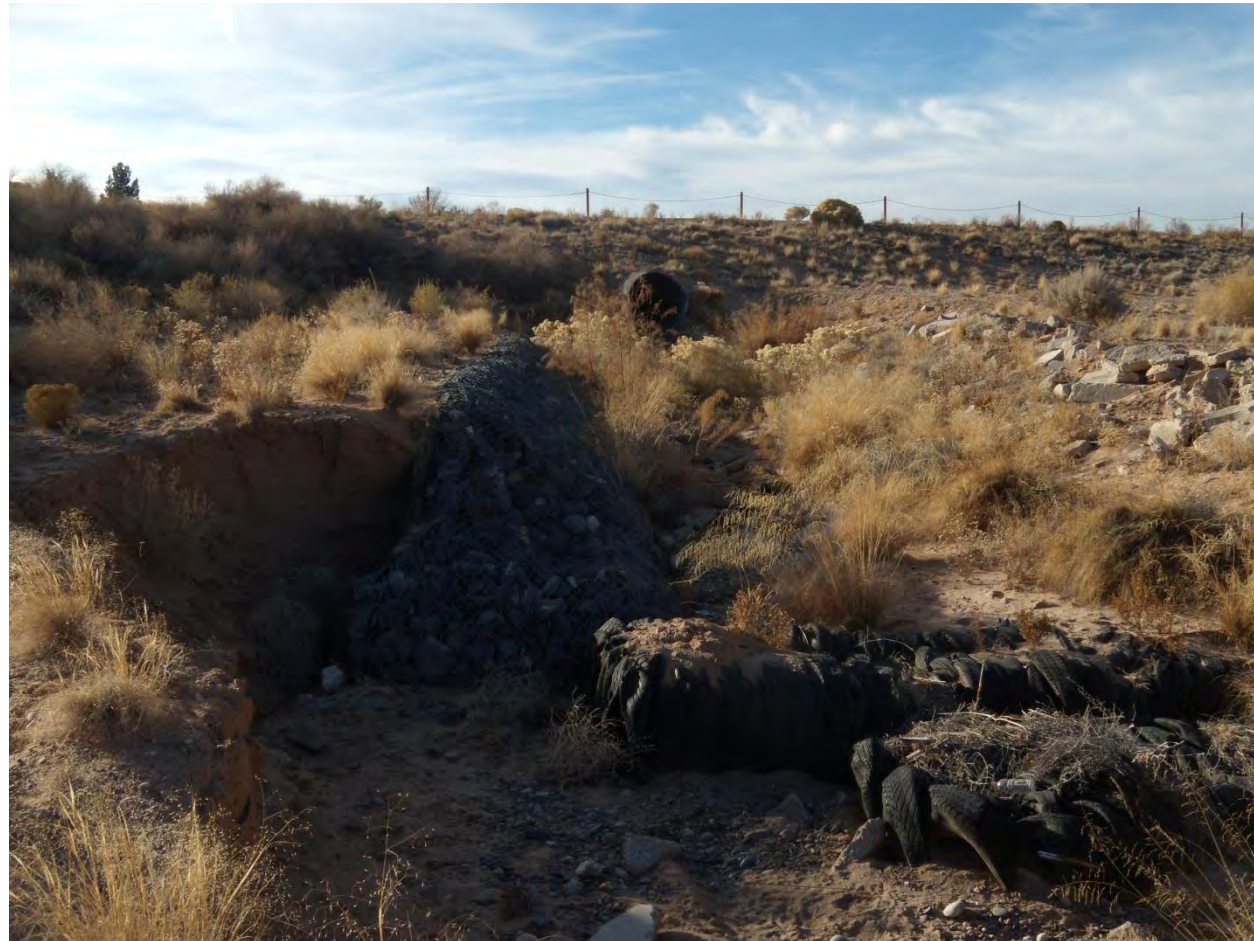
Photo 12: Failing tire bale drop structure downstream of Willow Creek Road.
