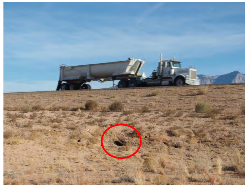
Photo 7: 30" CMP culvert under PDV, partially full of sediment.
