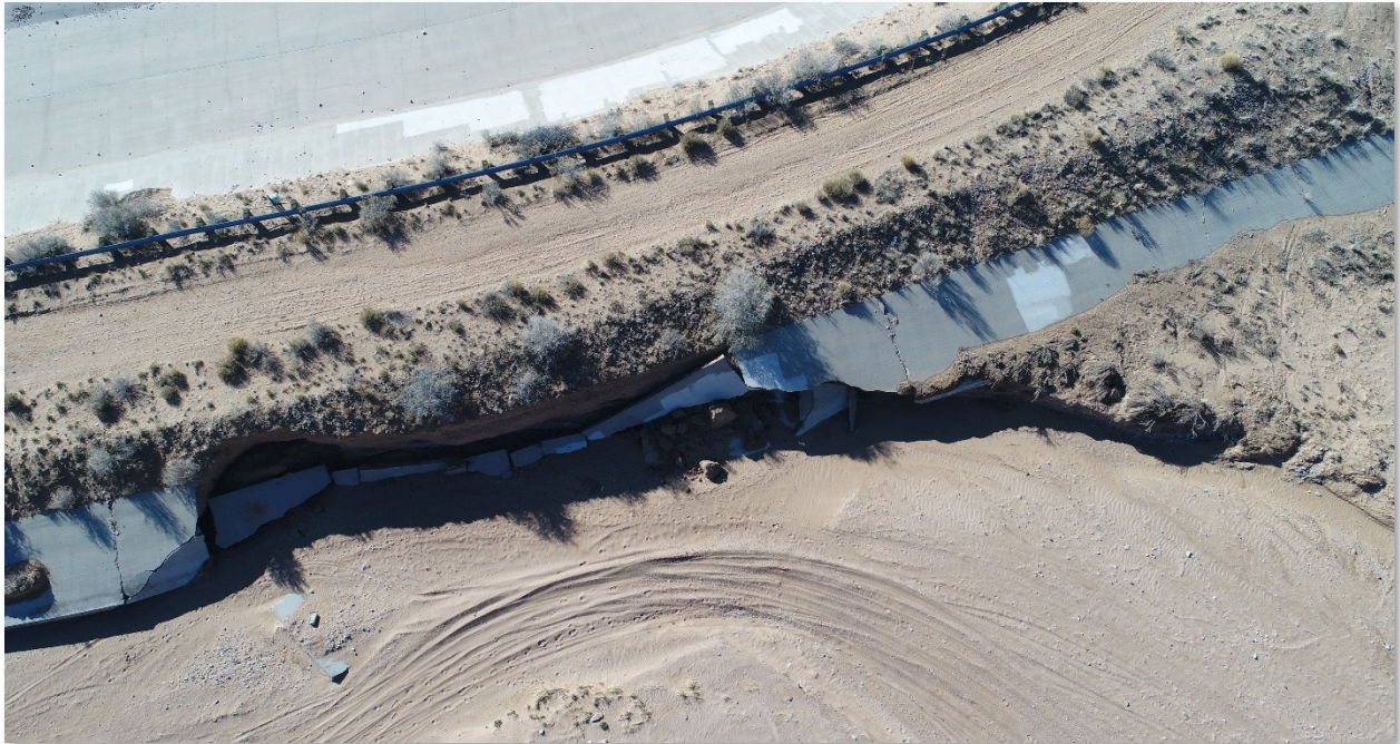
Figure 3.6: Failing bank protection in the lower Barranca Arroyo.
