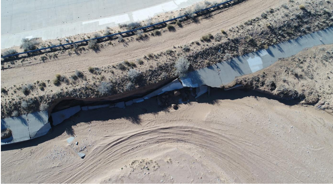
Figure 9: Concrete-lined Bank Failure Due to Erosion & Degradation
