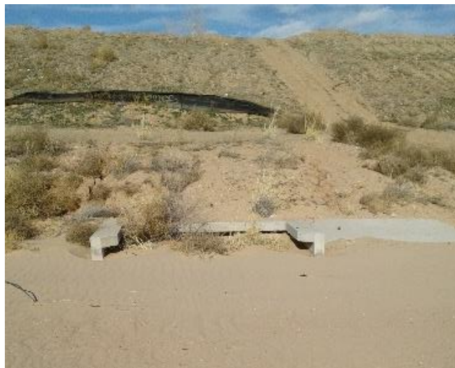
Figure 5: Buried Energy Dissipator in an Aggraded Channel
