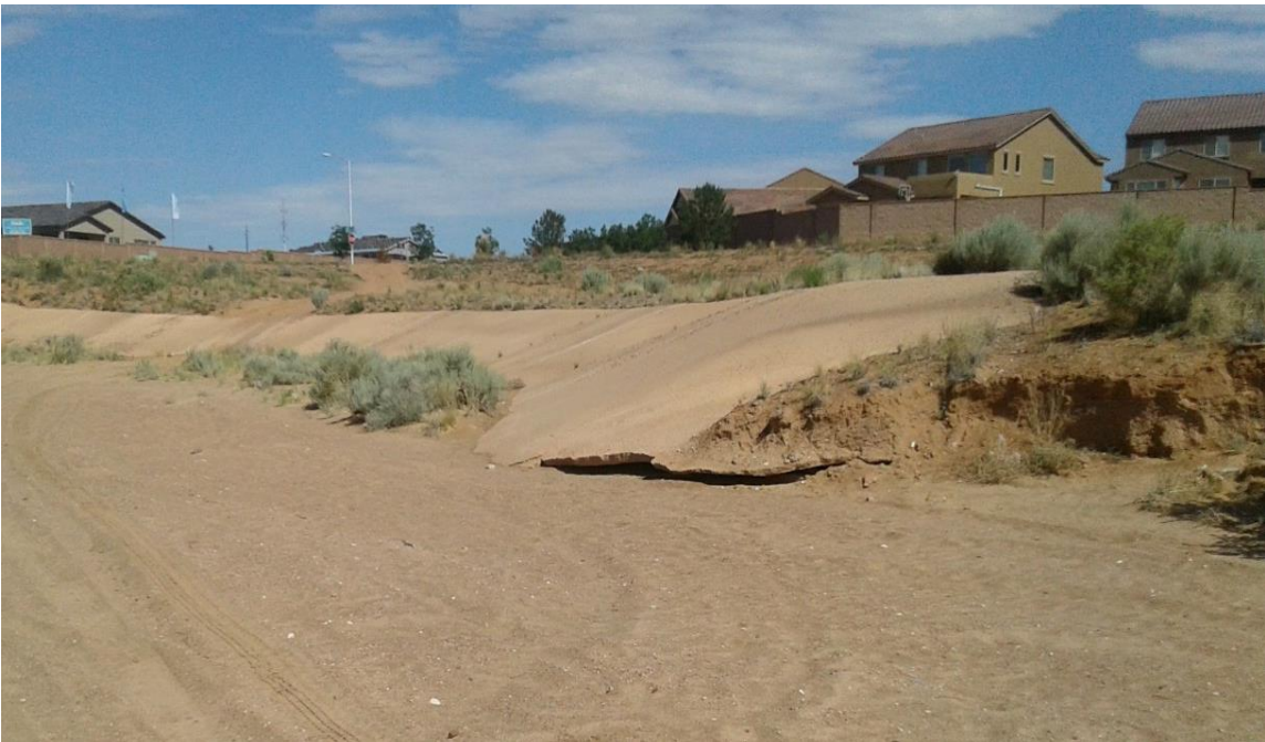
Figure 10: Shotcrete-lined Bank Failure Due to Erosion & Degradation
