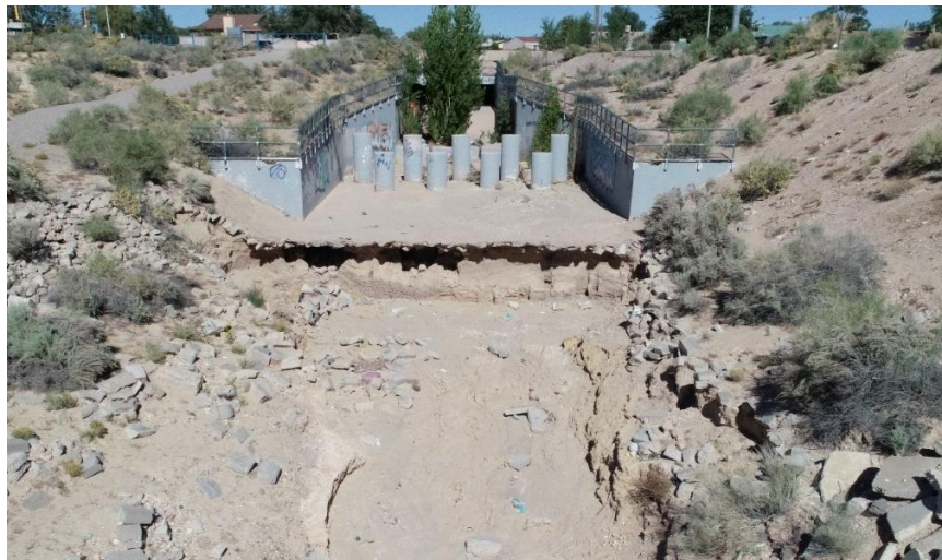
Figure 6: Loss of Sediment in a Degraded Channel
