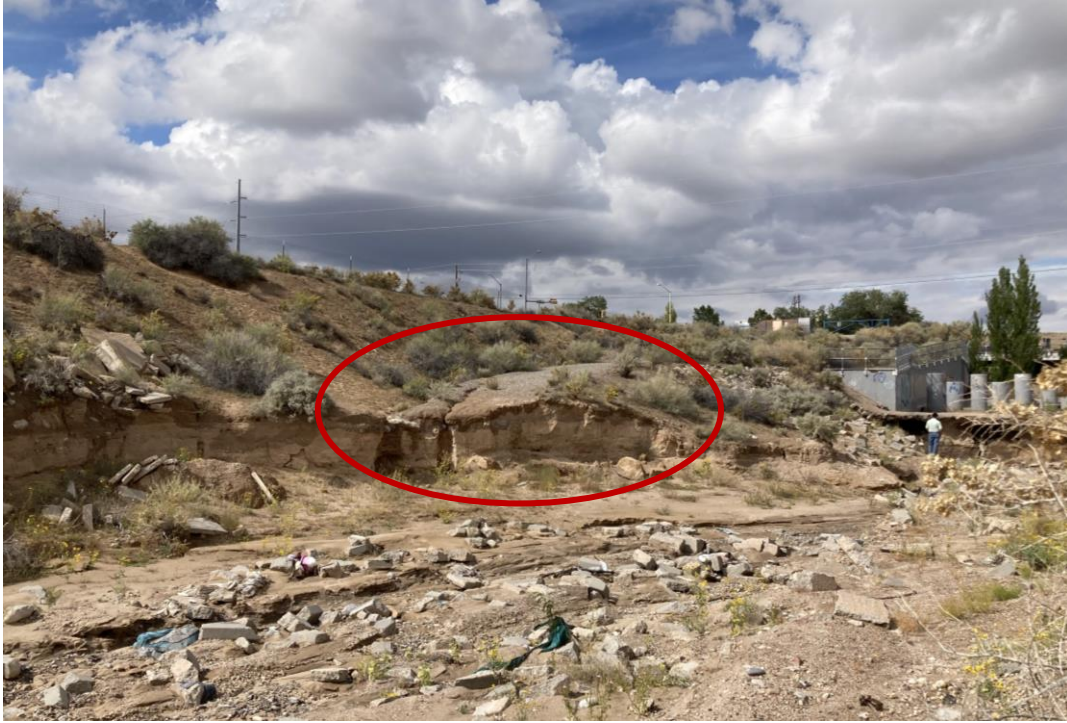
Figure 2: Channel Degradation & Damaged Maintenance Access Ramp.
